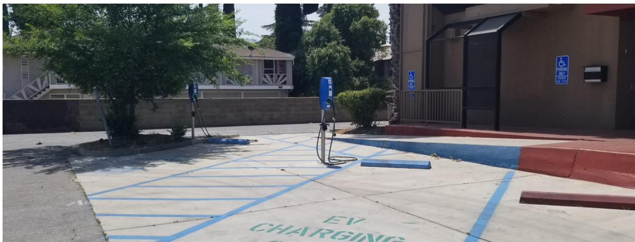
A Green Commuter EV charging installation at Fagbule Glass House Event Center in Fresno.
