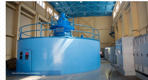
Holm Powerhouse Generators
